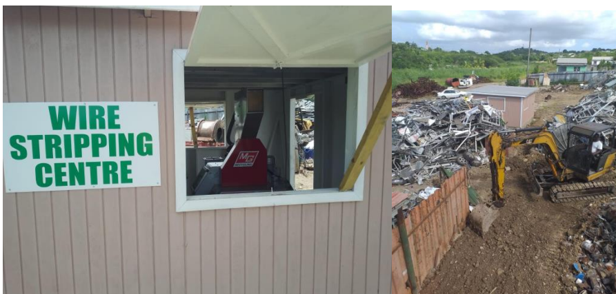
Photo 3. Tracking the land to plant underground wire to supply power to the wire stripping centre
