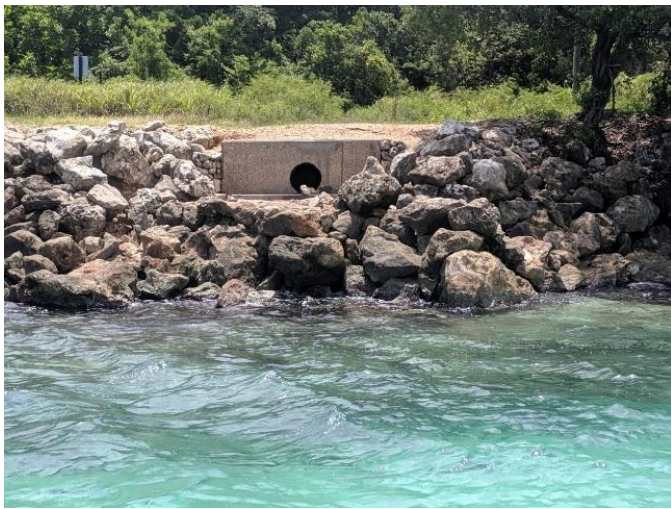
Photo 7. Old Folly Road Drain
